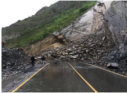
Fig. 3: The rockfall on the roadway.
